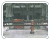
A-60 for PIPE & CABLE
